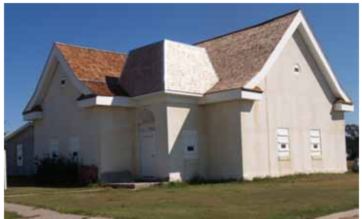
Watertight and stabilized, thanks to Price Construction Company and a cooperative agreement with NPS, September 2006!
