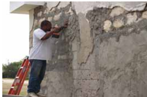
Assisting Mr. Price with some final stucco patching was subcontractor Charlie Scott, owner of DSK Drywall & Stucco of Hosington, Kansas. August 2006.
