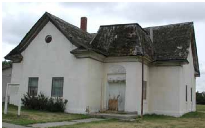
The Church as it appeared before work began in October 2005. There were major holes in the roof, birds were nesting in the eaves and inside the church, and the bell tower was about to collapse.
