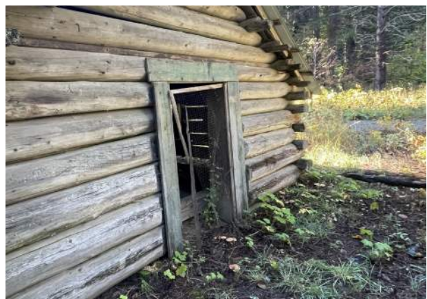
Image 43: The north elevation door opening is not secured. Wire mesh in wood frame broken.
