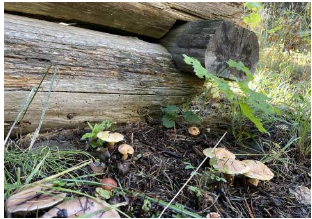
Image 32: The northwest corner of the cabin is sinking into the ground.
