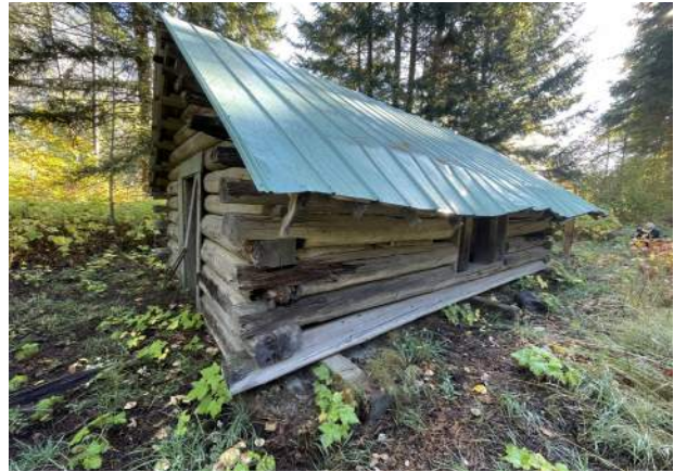
Image 35: The cabin does not have a foundation.
