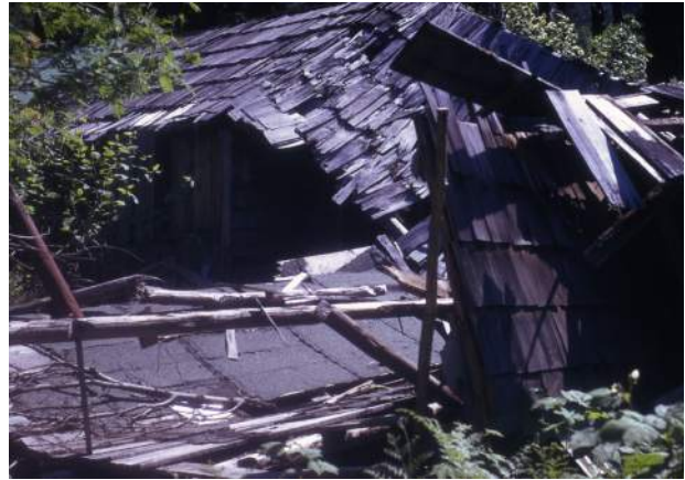
Image 7: Collapsed Courtney addition documented in 1973. NPS, North Cascades NPS Complex Museum Collection, NOCA 21818-282.
