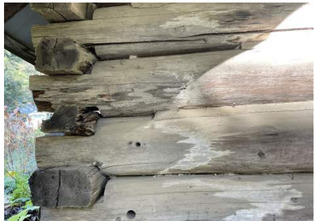
Image 33: Water staining on the south elevation.
