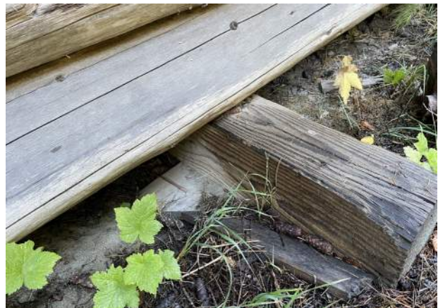
Image 36: Pressure treated sleepers are used to keep the building off the ground,
