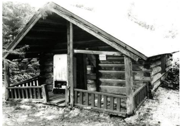
Image 55: Porch assembly in poor condition captured in 1984. National Park Service, North Cascades NPS Complex Museum Collection, NOCA 17312-57.
