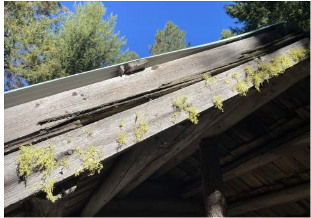
Image 25: Biogrowth present on south elevation fascia board.
