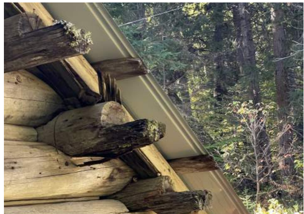
Image 23: Purlin ends on the north elevation are exposed.
