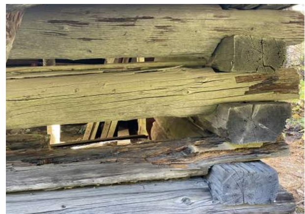
Image 28: Wall logs are severely deteriorated in locations, as seen here at the southwest wall corner.
