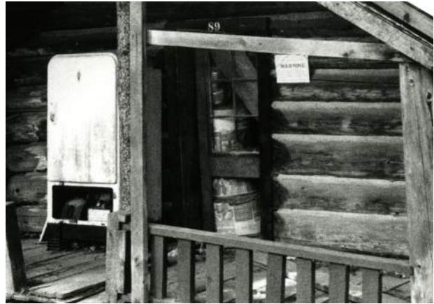
Image 53: Partially dismantled south door missing bottom panel at the Courtney Cabin captured in 1984. National Park Service, North Cascades NPS Complex Museum Collection, NOCA 17312-57.
