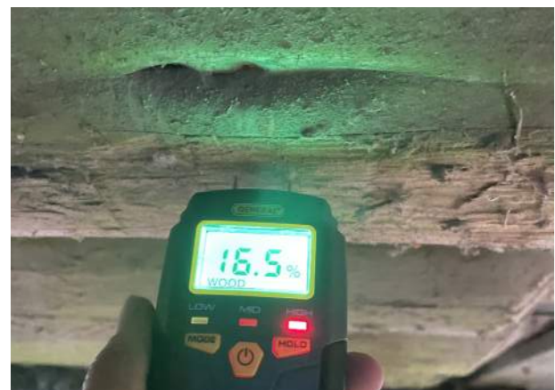
Image 47: Interior logs have high moisture content.
