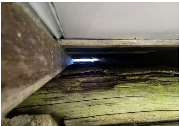
Image 21: The metal roof superstructure sits on wood purlins. Shakes are deteriorated.
