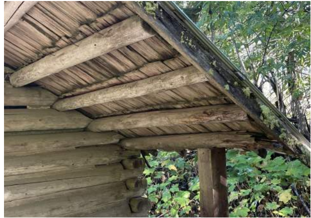
Image 22: The east most purlin is severely deteriorated and collapsing.
