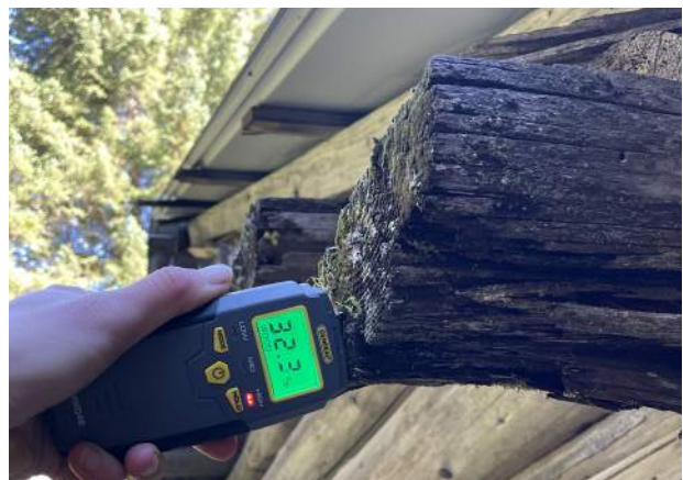
Image 24: Uncovered purlin ends have high moisture content.
