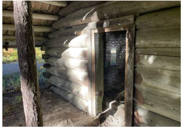
Image 41: The south door opening is secured with wire mesh in wood frame.
