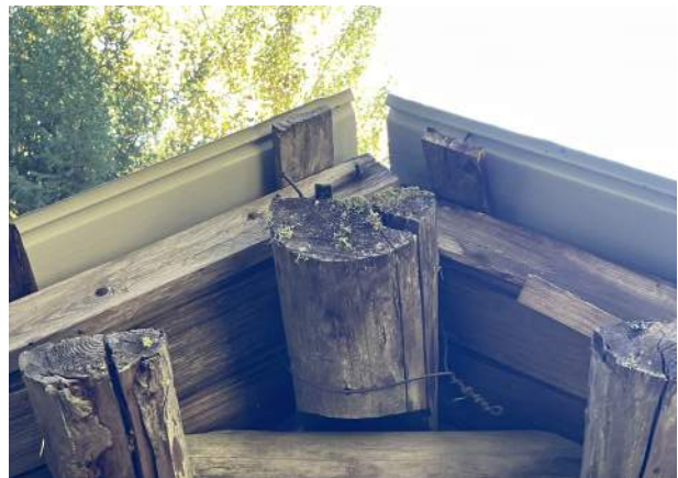
Image 20: The temporary metal roof is missing a ridge cap, allowing water to enter the roof system.
