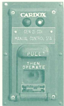
Nameplates on original generating unit 21, dating from 1925, in Gorge Powerhouse (WA-24-B-10).
