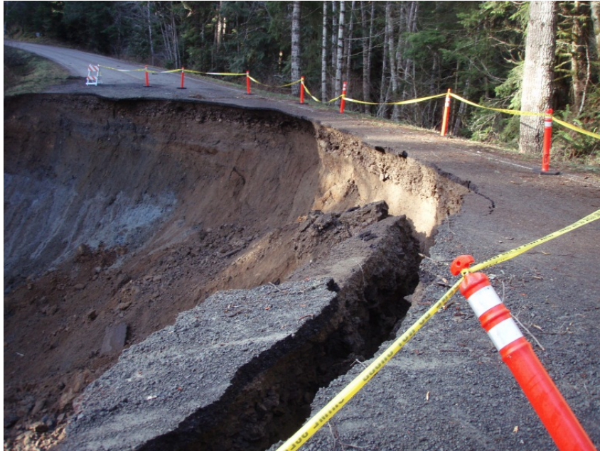
Figure 13. Slope failure destroyed the Hurricane Ridge Road in early January, 2010.
