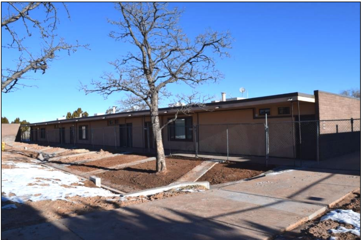
Photograph 26. Residence block B (Resource 14), south and east walls, with carport (Resource 18) at far left, with 2016 drainage improvements in foreground.
