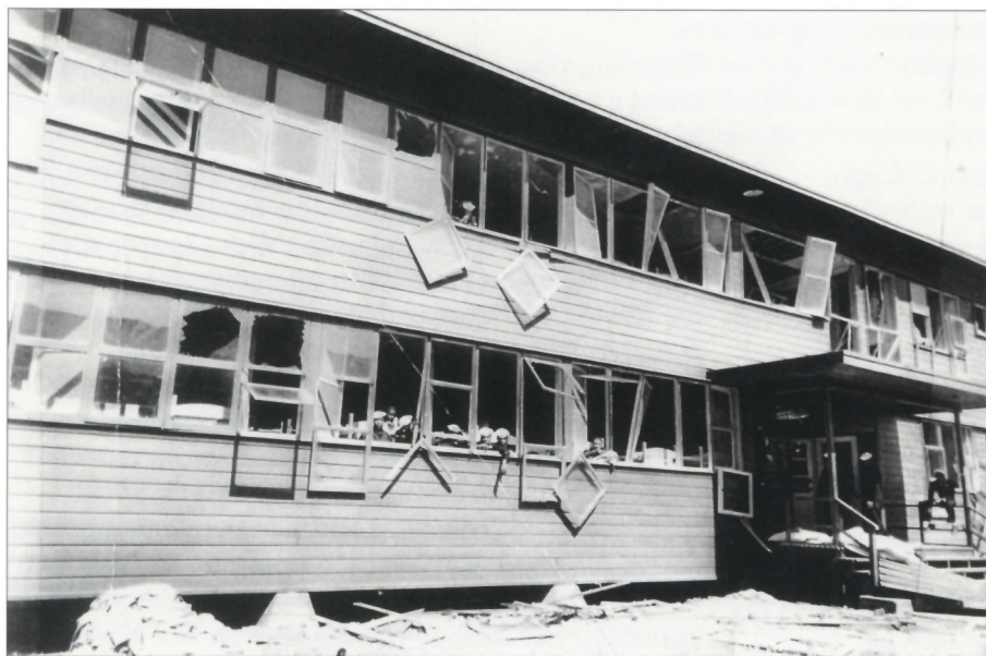
Barracks after explosion.
