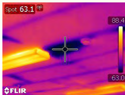
Insulation deficiency in fire building.
