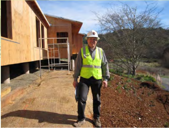
Construction Inspector Allan Lavery checking on the daily progress of the new hostel project.
