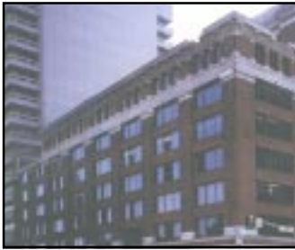
Prior to rehabilitation the building had inappropriate modern windows.
