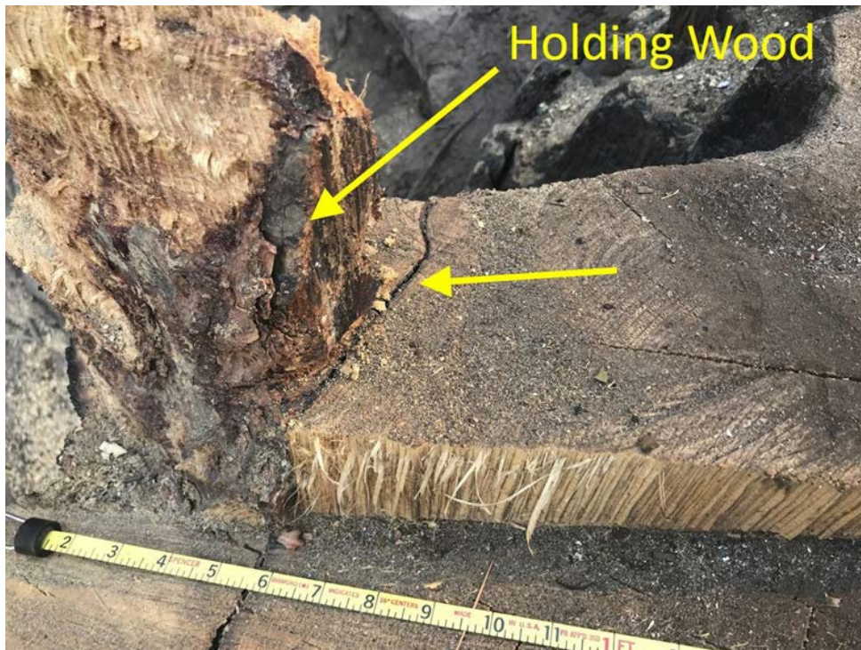
Figure 15: Arrows indicate an old fire scar showing bark inclusion within offside holding wood corner.
