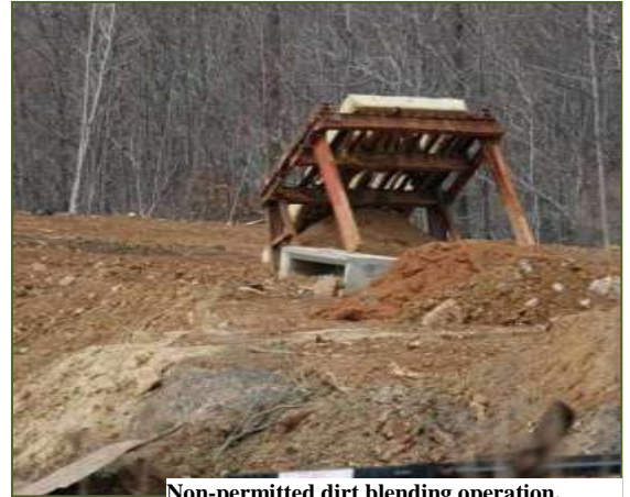
Non-permitted dirt blending operation.
