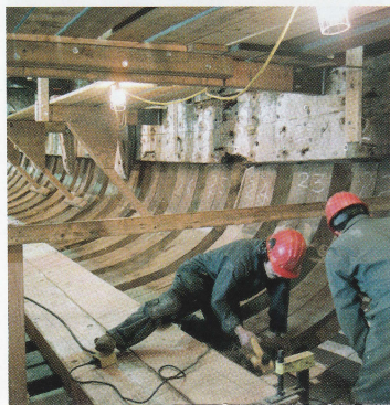
Workers prepare to install an 8-inch “thick ceiling” plank inside the hold. Some of these planks were 80 feet long, and all were tight-grained clear fir, as good as the original planking.
