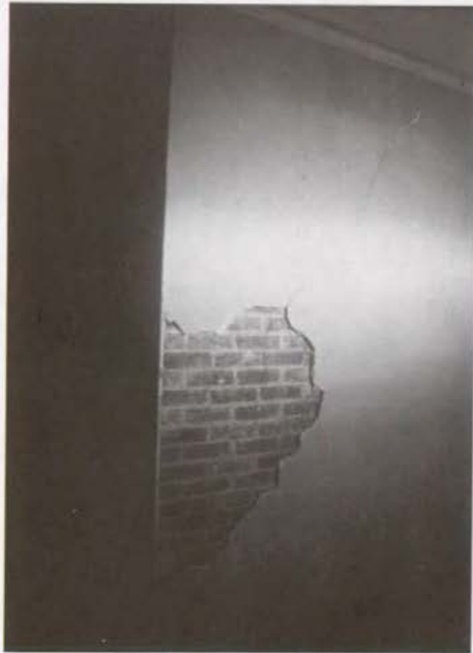
Alice's Room: Plaster Damage
