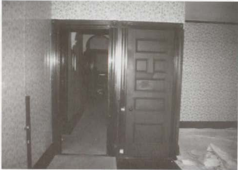
Typical Condition of Stained Woodwork
