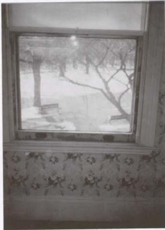
Typical Window Sash Condition Before Restoration
