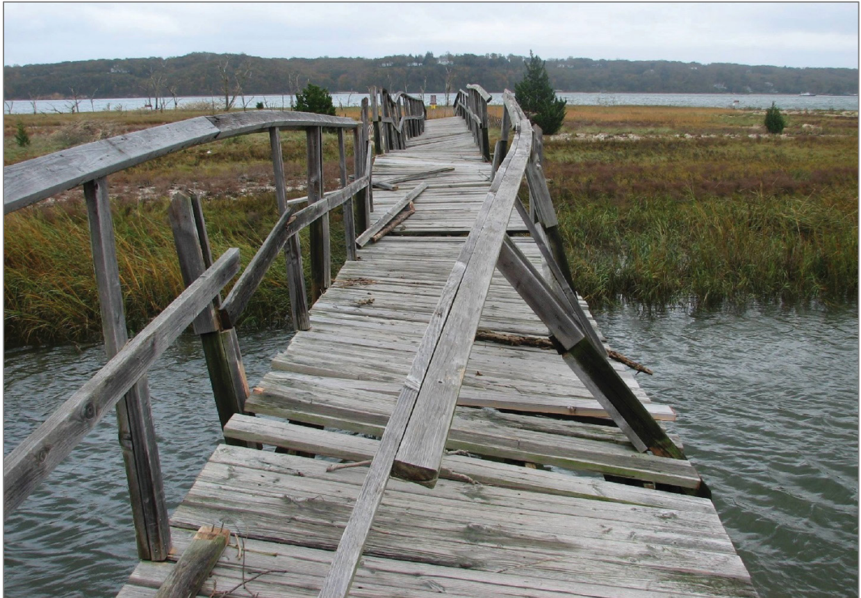
Figure 15. Photograph of damage to the nature trail boardwalk following Hurricane Sandy in October 2012. The sustained winds and storm surge of Hurricane Sandy irreparably damaged the 111 m (366 ft)-long boardwalk and limited visitor access to the Eel Creek wetland and Cold Spring Harbor beach. Destructive storm activity is a primary coastal management concern for the historic site. A single storm event such as Hurricane Sandy can significantly impact lowland regions, including the historic site's coastal geomorphology, habitats, resources, features, and infrastructure. (NPS/SAGAMORE HILL NATIONAL HISTORIC SITE).
