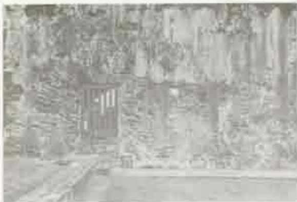
Figure 8. San Cristóbal, north wall of ramp leading to Main Gate. (Photo by J. Restonitz, 1998.)
