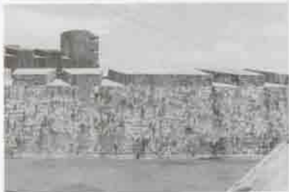
Figure 10. San Cristóbal, exterior wall of North Section. (Photo by J. Jacob, 1989.)
