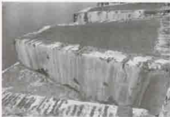
Figure 23. Santa Barbara Battery, sections on the south side. (Photo by J. Jacob, 1989.)
