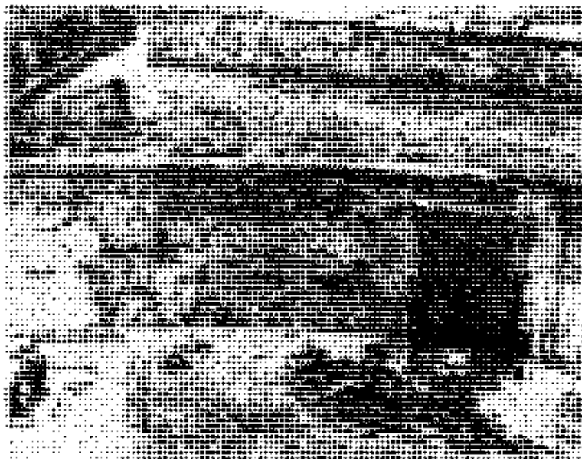
Figure 12.26. APW photo showing work on the curved covered way, May 1963. (San Juan NHS Archives.)
