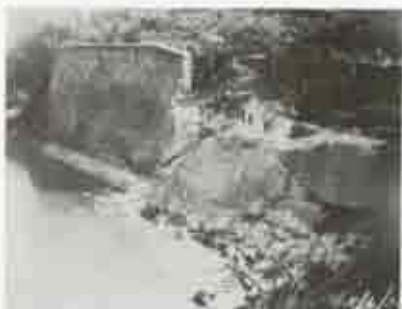
Figure 17. Workers beginning to work on the collapsed curtain wall between Santa Elena and San Agustín. [West Wall], 1938. (SAJU NNS Archives.)
