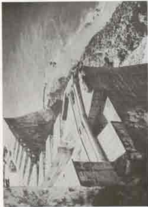
Figure 19. World War II search light trunk at the east end of Santa Barbara Station demolished. (P.O. Gjessing, 1957, pack files.)
