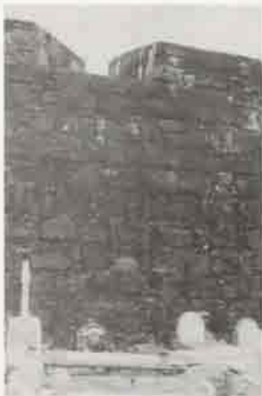
Figure 1. North wall of San Juan, backing cemetery. Note use of ashlar with stone chinking (this wall has more chinking than other walls); brick chinking and brick of merlons may be repairs. Photo by J. Jacob, 1949.
