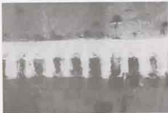
Figure 3. Casted hollow brick along banquette on south side of Santa Barbara Battery. 3. Decorative brick-dust stucco partially remains, covering brick faces. Photo by J. Jacob, 1989.
