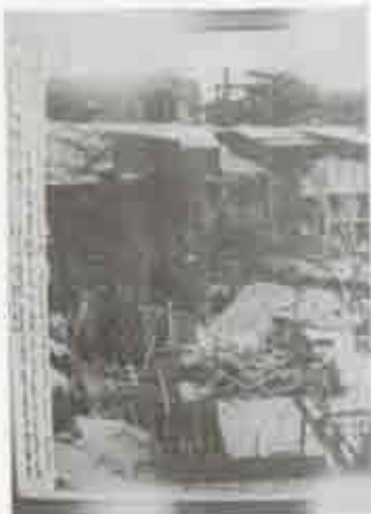
Figure 29. New concrete foundation at NW corner of San Agustín Station. [West Wall], 1938. (SAJU NHD Archives.)
