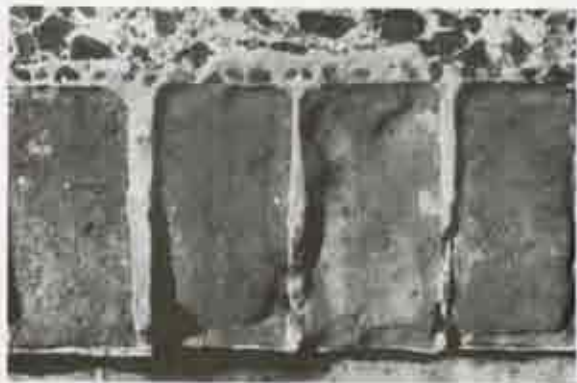
Figure 4. Northwest edge of ramp connecting the Plaza de Armas and Santa Barbara Battery. Brick galling is located between brick and bossing. Photo by J. Jacob, 1989.
