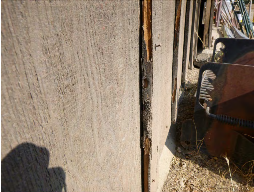
Impacts 7: Termite damage on Mill/Carpenter Shop (NPS, August 2021).
