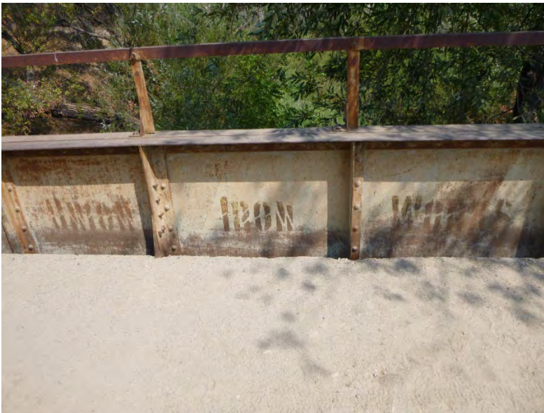
Impacts 10: Rusting metal on Medea Bridge (NPS, August 2021).
