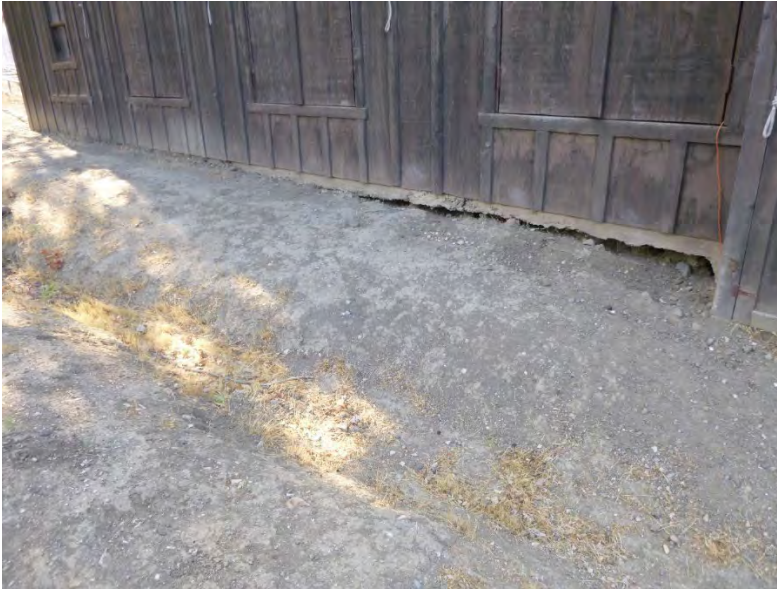
Impacts 9: Eroded foundation at Mill/Carpenter Shop (NPS, August 2021).
