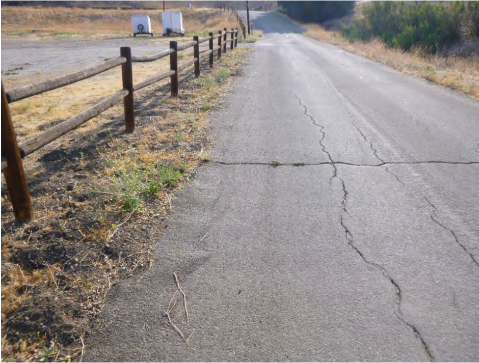
Impacts 5: Cracking asphalt in Original Entry Road (NPS, August 2021).
