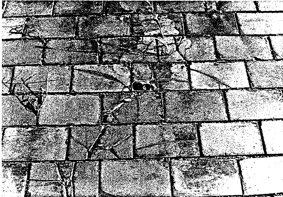
2.1 Passageway. Loose and cracked roof tiles on Section A.
