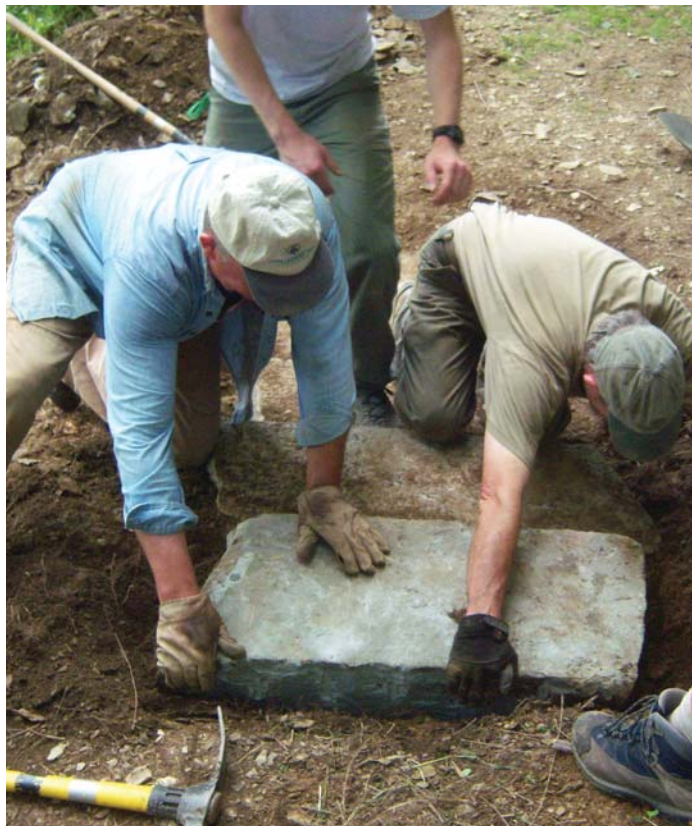
PATC crews prepare the route and foundation for the Stone Steps from the Appalachian NST up to the Lockwood House. NPS photo.
