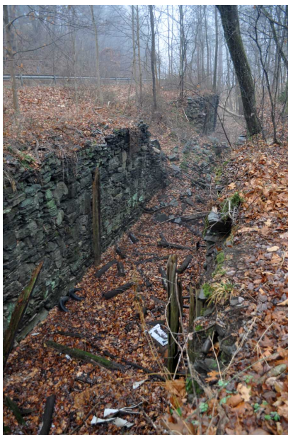
Collapsed wall at Lock 71 with Route 79 in background.
