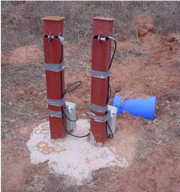
Figure 7. Photo of Wells WB-07 and WB-08, showing standpipe completion and transducer installation (2003).
