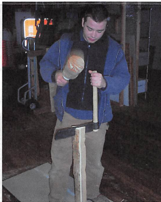
Hand-splitting each picket using a froe and mallet creates a rustic yet controlled cut. PTEI photo.
