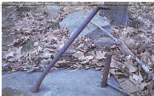
In certain areas the iron brace supports were all that was left of the original fence material.
