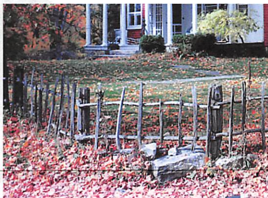
The existing fence was dilapidated and no longer looked the way it did when it was first built.
