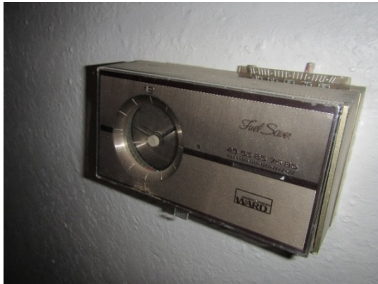
Figure M03. Pellet burner thermostat in Living Room 100. (HEI 2015)
