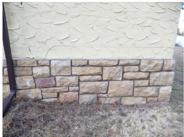
Figure X16. South Elevation horizontal crack detail at porch floor. (SRJA 2015)
