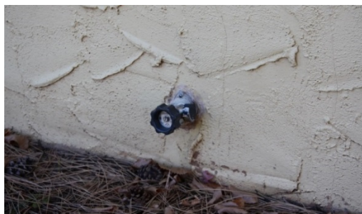
Figure P04. Wall hydrant. (SRJA 2014)
