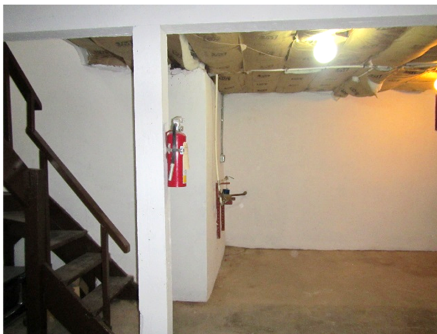
Figure F01. Fire extinguisher in Basement 001 (HEI 2015)
