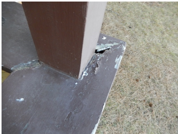
Figure X8. Porch northeast column and wall cap deterioration. (SRJA 2015)
