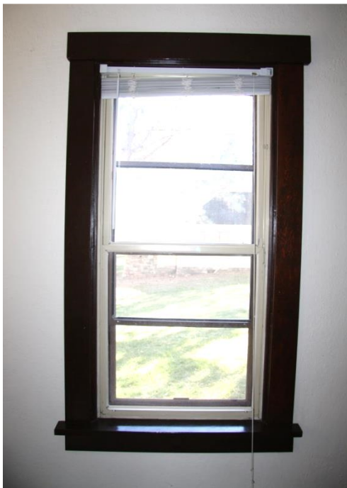
Figure W7. Detail of inappropriate aluminum interior replacement Window 103. (SRJA 2014)
