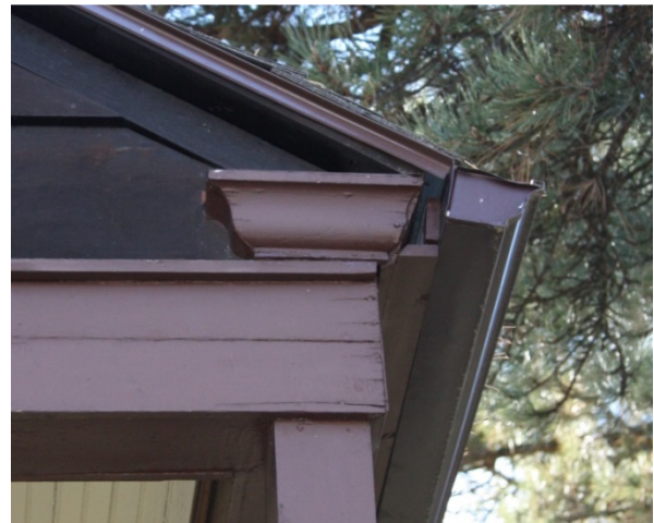
Figure X10. Northeast corner of porch gable. From this angle, the wood cornice on the north side of the house appears to have been replaced with a flat trim board. This detail is not very noticeable. (SRJA 2014)
