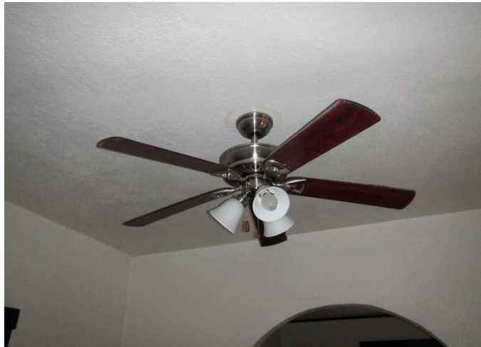
Figure E07. Ceiling fan located in Dining Room 101. (HEI 2015)
