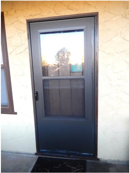
Figure X11. Door 100/1 Aluminum storm door. Note the weatherstripping at the base has become detached and requires repair or replacement. (SRJA 2014)
