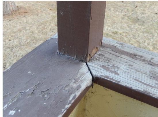
Figure X9. Porch southeast column and wall cap deterioration. (SRJA 2015)
