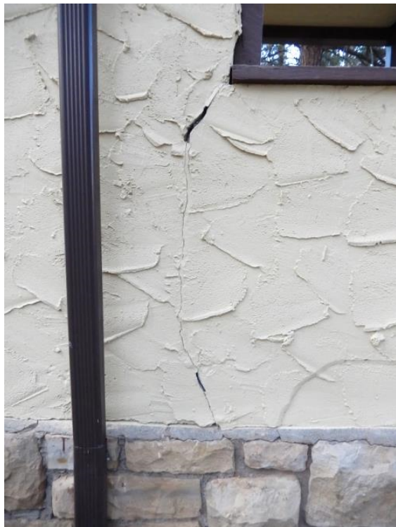
Figure X15. South Elevation crack detail at porch. (SRJA 2015)
