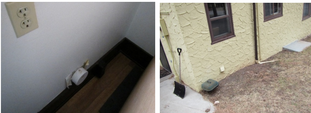
Figure M07. Mud Room 107, Dryer vent and termination. (HEI 2015)
