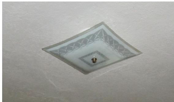
Figure E11. Light fixture located in Bedrooms 106, 107, and 109. (HEI 2015)
