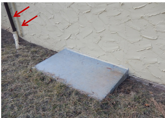
Figure X19. South Elevation basement Window 001. The exposed pipe on the left is the downspout. The painted pipe on the right is the exposed kitchen sink vent pipe. (SRJA 2015)
