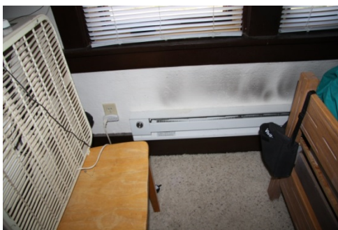
Figure 1-34. Bedroom 106 Looking east. Note the staining on the wall above the baseboard heater. (SRJA 2014)
