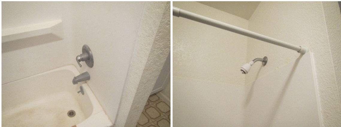
Figure P12. Shower in Bathroom 108. (HEI 2015)
