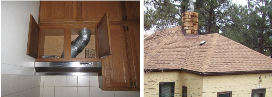
Figure M06. Kitchen 102, Exhaust hood and termination. (HEI 2015)
