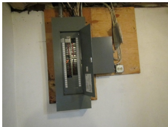
Figure E04. Electrical panel located in Basement 001. (HEI 2015)
