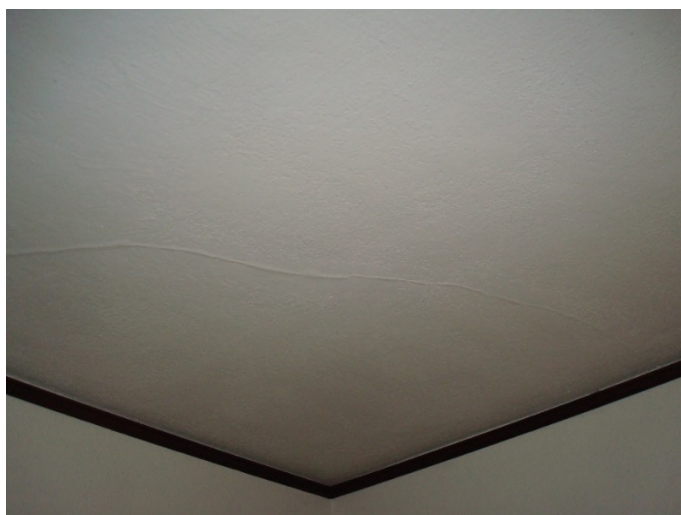
Figure S7. Crack in ceiling of room 100. (SEA 2015)
