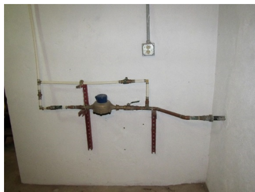
Figure P06. Domestic water entry in Basement 001. (HEI 2015)
