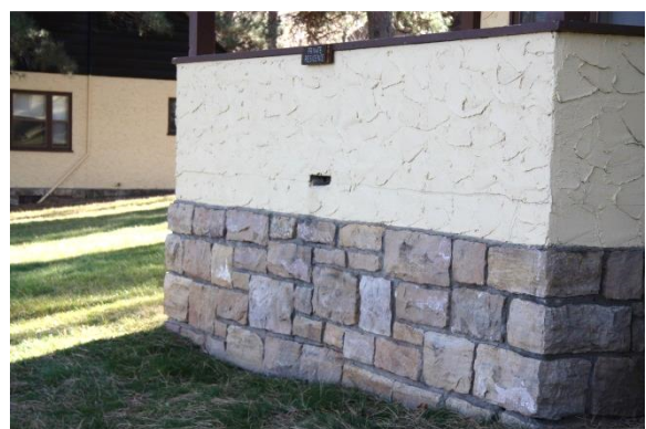
Figure X6. Porch east wall detail with cracking at floor level. (SRJA 2015)
