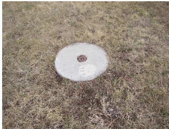
Figure P02. Exterior shutoff valve for water system. (HEI 2015)
