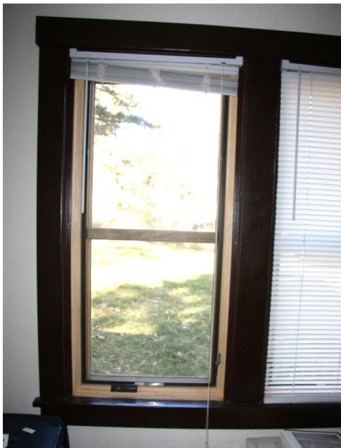
Figure W11. Detail of inappropriate aluminum interior replacement Window 113. (SRJA 2014)
