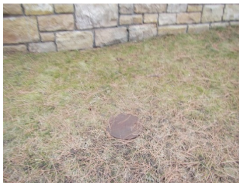
Figure P07. Sanitary sewer cleanout in east yard. (HEI 2015)
