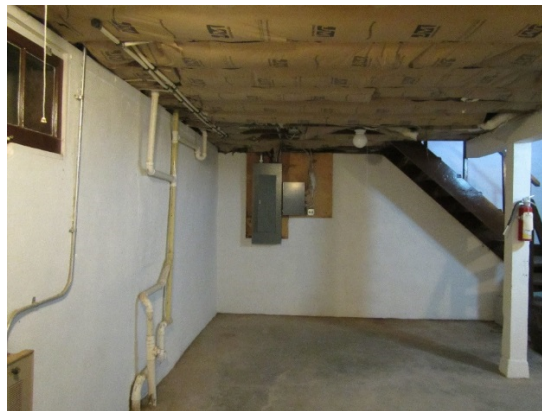
Figure E03. Electrical service panelboard located in Basement 001. (HEI 2015)
