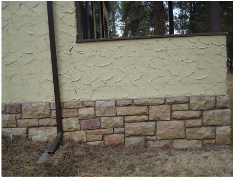
Figure S9. Crack in south wall. (SEA 2015)
