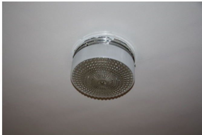
Figure E08. Light fixture located in Kitchen 102. (SRJA 2014)
