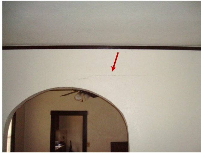
Figure S5. Crack over Door 100/2. (SEA 2015)
