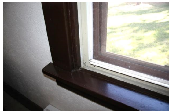
Figure W8. Detail of inappropriate aluminum interior replacement window with exterior brown storm window at Window 103. (SRJA 2014)
