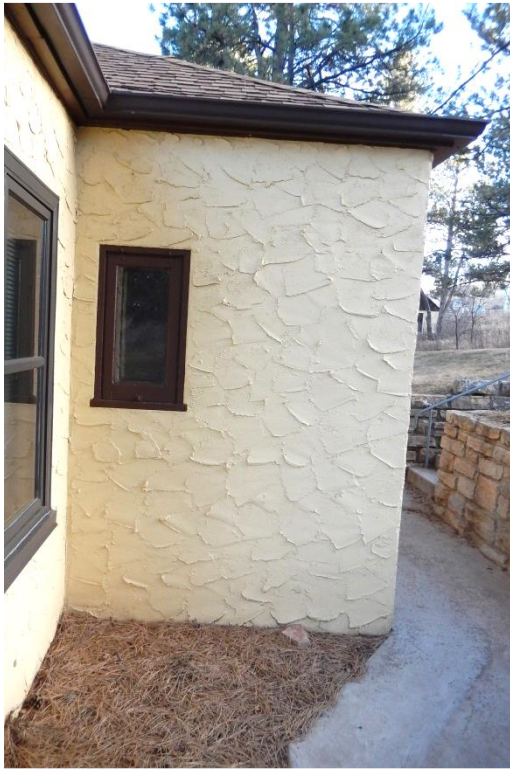
Figure X32. North Elevation Window 108. Note the grade is above the top of the stone foundation wall (SRJA 2015)
