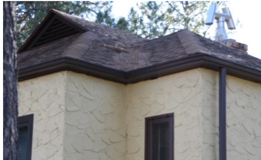
Figure R1. Valley and gutters filled with pine needles. (SRJA 2014)
