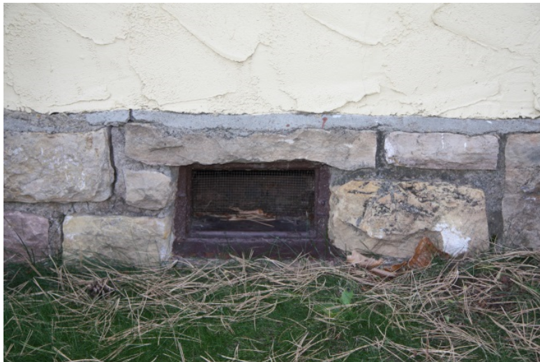
Figure X34. North Elevation crack detail east of foundation vent. (SRJA 2015)
