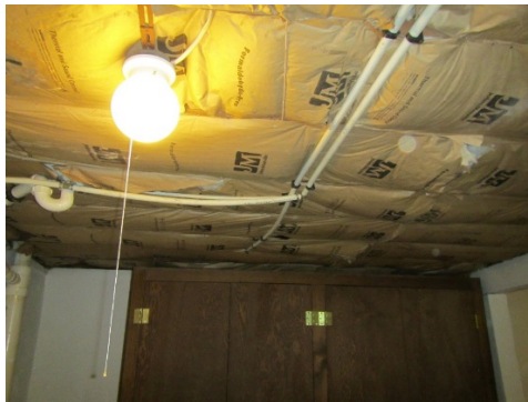
Figure E05. Light Fixture located in Basement 001. (HEI 2015)
