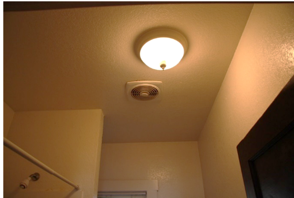
Figure E12. Light Fixture located in Bathroom 108. (SRJA 2014)
