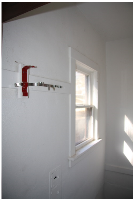
Figure 1-27. Stair 104 west wall. Note the old fuse panel that is no longer used. (SRJA 2014)
