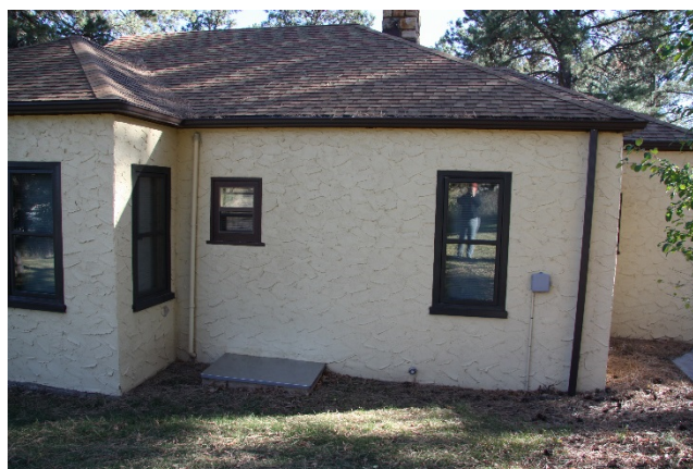
Figure E14. Telephone service entrance located on the north exterior of the house. (SRJA 2014)
