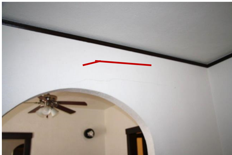
Figure 1-9. Living Room 100 looking at crack in wall above Door 100/2. (SRJA 2014)
