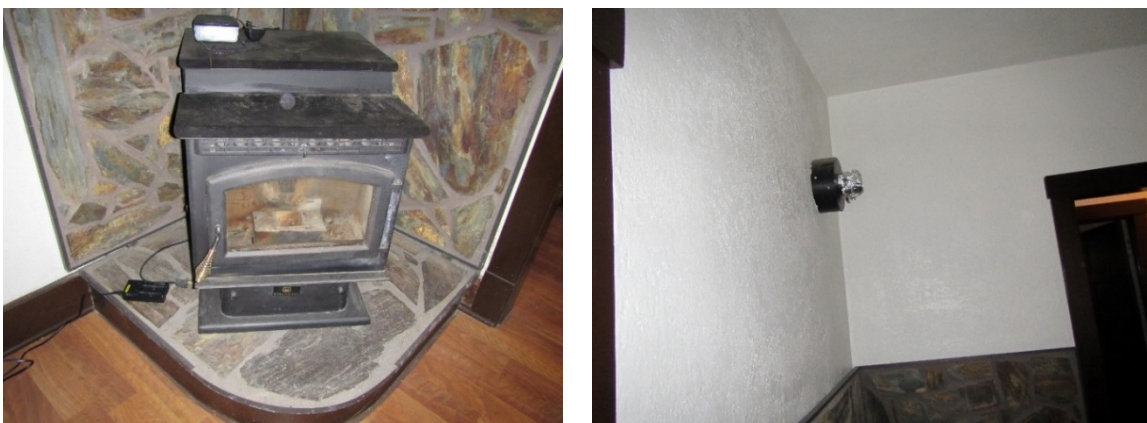
Figure M02. Dining Room 102, Pellet burner and capped flue. (HEI 2015)
