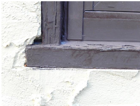
Figure X17. South Elevation detail of deteriorating wood trim at window and missing stucco at Window 106. (SRJA 2015)
