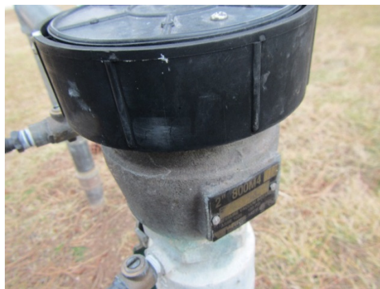
Figure P03. Irrigation vacuum breaker. (HEI 2015)
