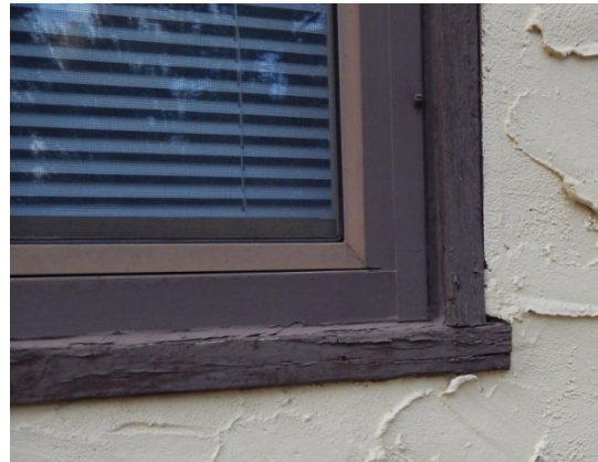
Figure W4. Detail of typical window trim deterioration where the historic trim is exposed. This shows signs of many peeling paint layers and wood rot at Window 103. (SRJA 2015)
