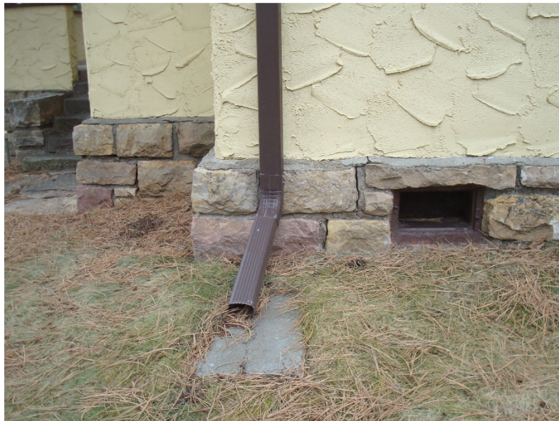
Figure S10. Crack in foundation, north elevation. (SEA 2015)
