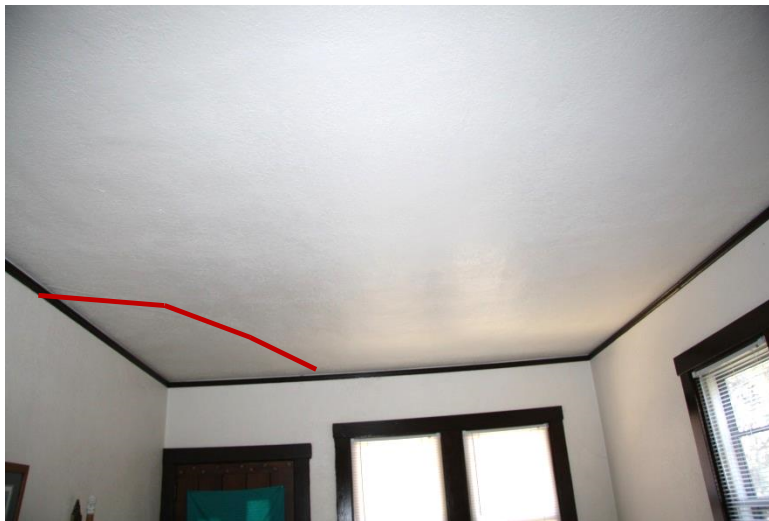
Figure 1-10. Living Room 100 looking at cracks in ceiling. (SRJA 2014)
