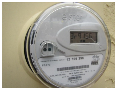
Figure E02. Exterior electrical service meter on the west side of the house. (HEI 2015)
