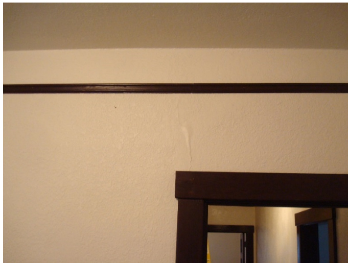
Figure S6. Crack over Door 109/1. (SEA 2015)
