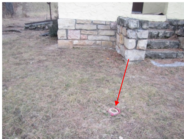
Figure P05. Damage exterior sanitary sewer cleanout. (HEI 2015)
