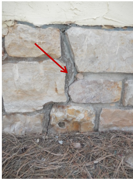
Figure X5. Porch – East Elevation foundation crack detail. The red arrow indicates a vertical crack through the mortar joints from below grade to the top of the foundation wall. (SRJA 2015)
