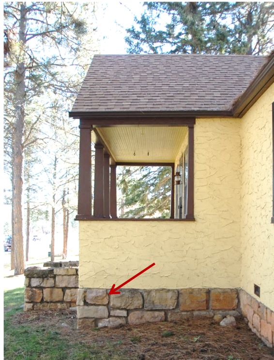
Figure X3. Porch - North Elevation. The red arrow identifies a crack. (SRJA 2014)
