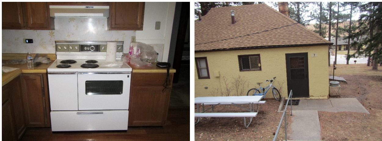
Figure M03. Kitchen 104, Exhaust hood and termination. (HEI 2015)
