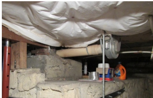
Figure M06. Radon system in Basement 005. (HEI 2015)
