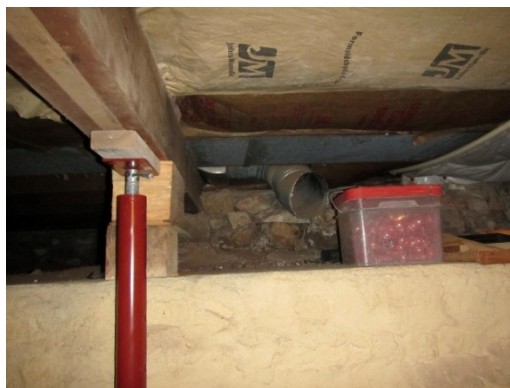
Figure M07. Example of abandoned ductwork in Basement 001. (HEI 2015)
