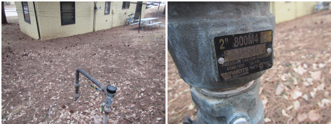
Figure P01. Irrigation vacuum breaker. (HEI 2015)
