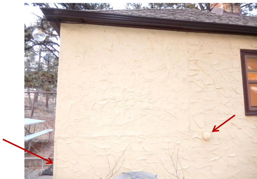
Figure X23. South Elevation at west side. Outline of infilled screen porch can be seen. The right red arrow points to a clean-out installed in the wall. The left arrow points to a large vertical crack at the corner. (SRJA 2015)
