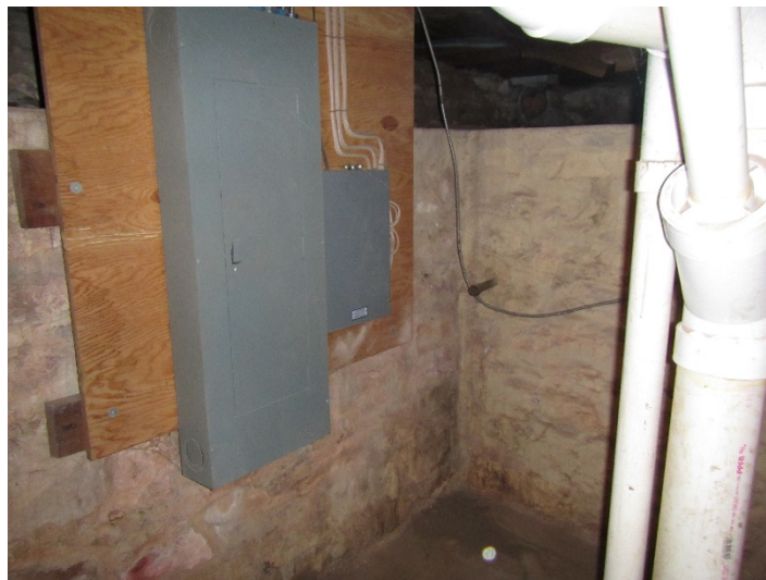
Figure E04. Electrical service panelboard located in Basement 001. (HEI 2015)
