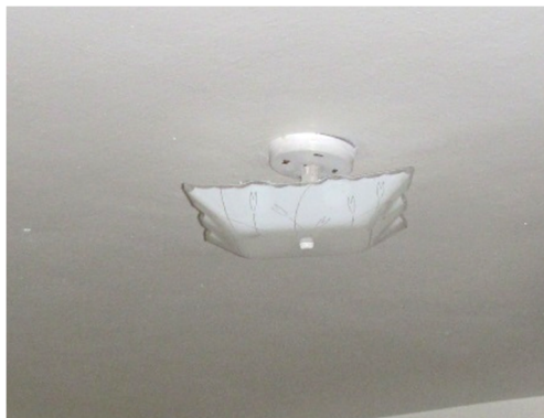
Figure E14. Light fixture located in Bedrooms 106 and 107. (HEI 2015)
