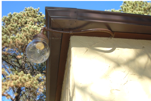
Figure X35. West Elevation exterior light fixture at southwest corner. (SRJA 2014)
