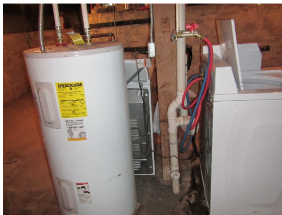
Figure P03. Domestic electric water heater in Basement 001. (HEI 2015)
