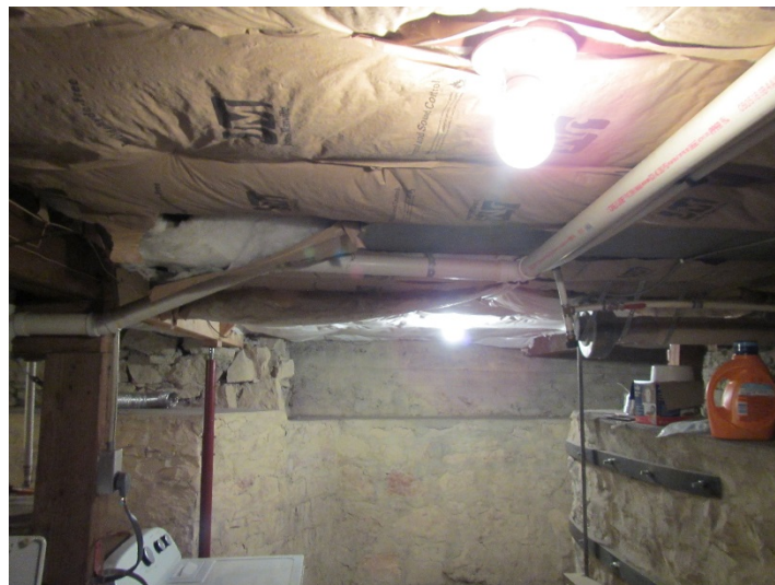
Figure E06. Light fixtures located in Basement 001. (HEI 2015)
