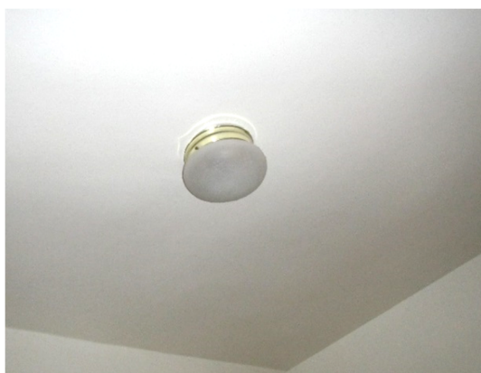
Figure E11. Light fixture located in Breakfast Nook 102. (HEI 2015)
