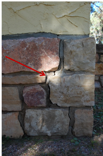
Figure X11. Porch - South Elevation crack detail. (SRJA 2014)
