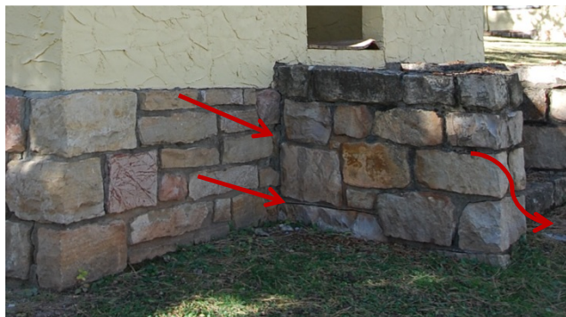
Figure X9. Porch – East Elevation and south wall of steps. The red arrows indicate open mortar joints due to wall movement. The curved arrow indicates the wall is beginning to rotate forward. (SRJA 2014)
