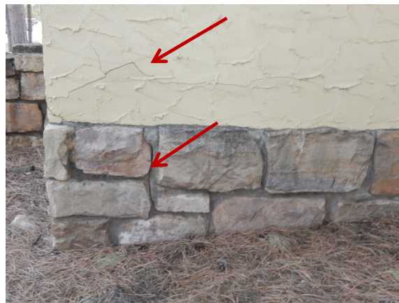
Figure X4. Porch – North Elevation foundation and stucco cracks. The top red arrow identifies a long traveling crack in the stucco. The bottom red arrow identifies a long vertical crack in the mortar joints that begins below grade and projects to the top of the foundation wall. (SRJA 2015)
