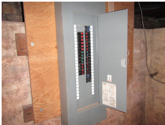
Figure E05. Electrical panelboard located in Basement 001. (HEI 2015)
