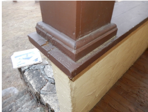
Figure X12. Porch – Center column detail with wood deterioration at bottom cap. (SRJA 2015)
