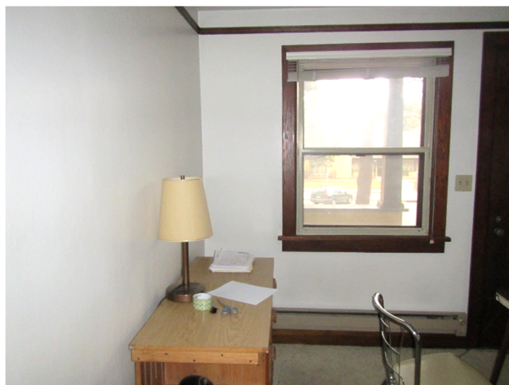
Figure M01. Example of electric baseboard heaters In Living 100. (HEI 2015)
