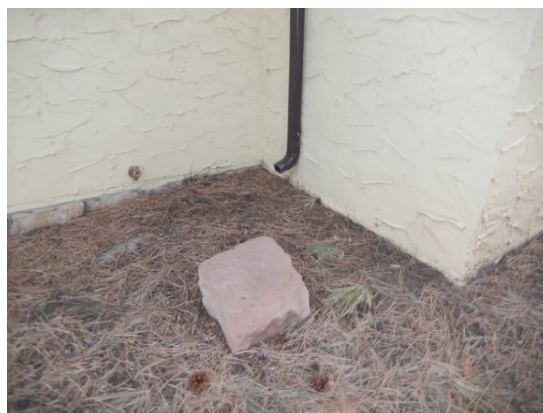
Figure X21. Northeast corner of the building. The grade is well above the top of the stone wall and the stucco is cracked and has peeling paint. The downspout extension is missing. (SRJA 2015)
