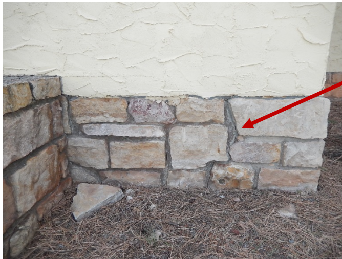
Figure S13. Crack in east foundation wall. (SRJA 2015)
