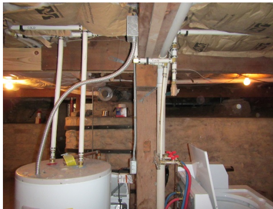
Figure P08. Washing machine connections in Basement 001. (HEI 2015)
