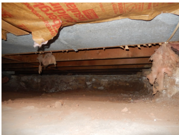
Figure B-14. Basement Room 001 Looking into north crawl space. Note the insulation is missing here. (SRJA 2014)
