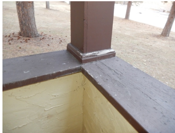
Figure X13. Porch – northeast column detail of missing paint. (SRJA 2015)
