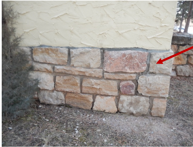
Figure S12. Crack in south foundation wall. (SRJA 2015)
