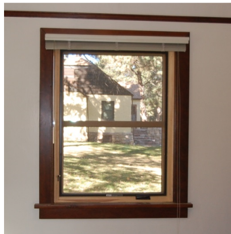
Figure W7. Window 108 replacement window that is not finished on the interior. (SRJA 2014)
