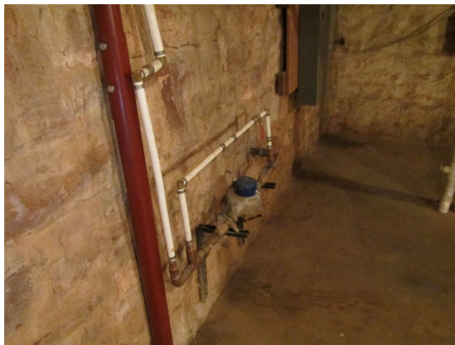
Figure P04. Domestic water entry in Basement 001. (HEI 2015)
