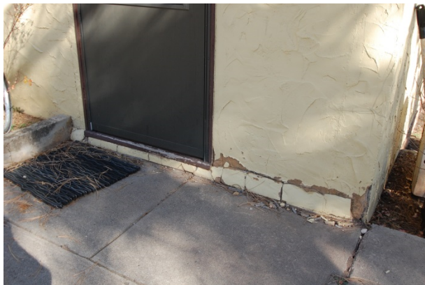
Figure X30. West Elevation. Showing concrete landing and stucco wall deterioration. (SRJA 2014)
