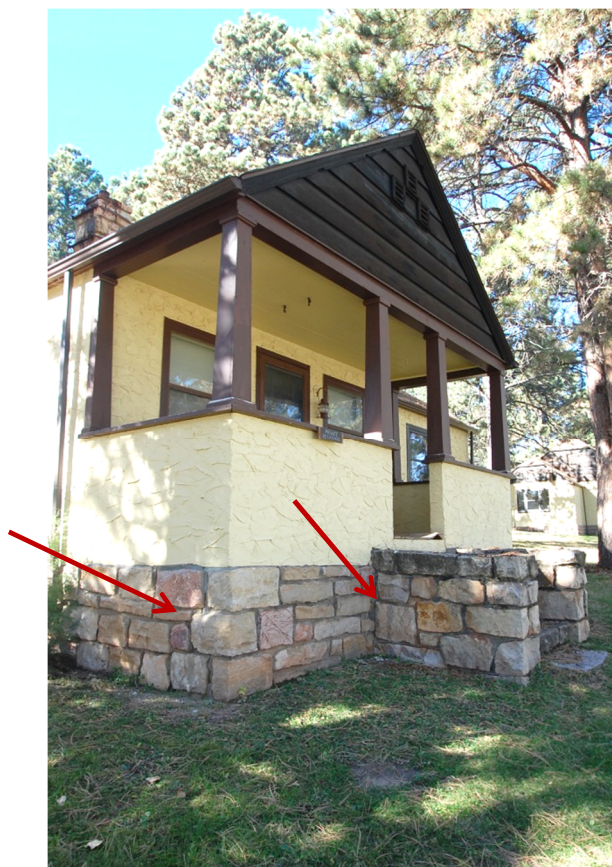
Figure X2. East porch. The red arrows identify cracks. (SRJA 2014)
