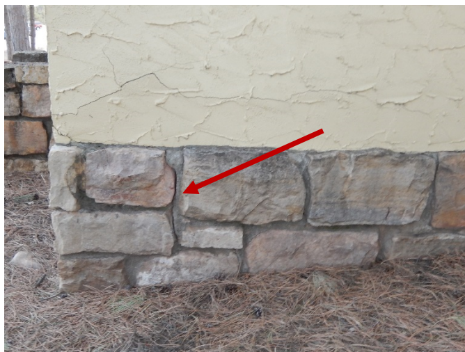
Figure S14. Crack in north foundation wall. (SRJA 2015)
