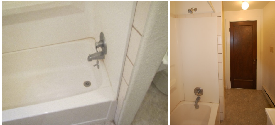
Figure P10. Shower in Bathroom 104. (HEI 2015-Left, SRJA 2015-Right)
