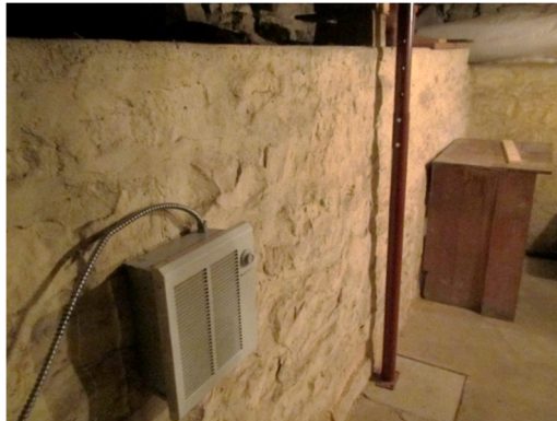
Figure M05. Electric heater in Basement 002. (HEI 2015)
