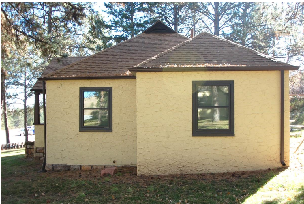
Figure X36. North Elevation. Note the grade is very high at the west side. The downspout extension is missing. (SRJA 2014)
