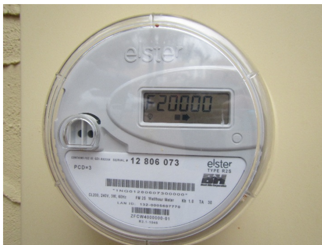
Figure E03. Exterior electrical service meter on the west side of the house. (HEI 2015)
