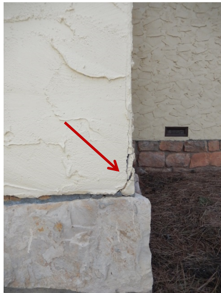
Figure X6. Porch – East Elevation stucco crack at northeast corner. The red arrow identifies a crack in the corner of the plaster that has traveled from the north side of the wall. (SRJA 2015)
