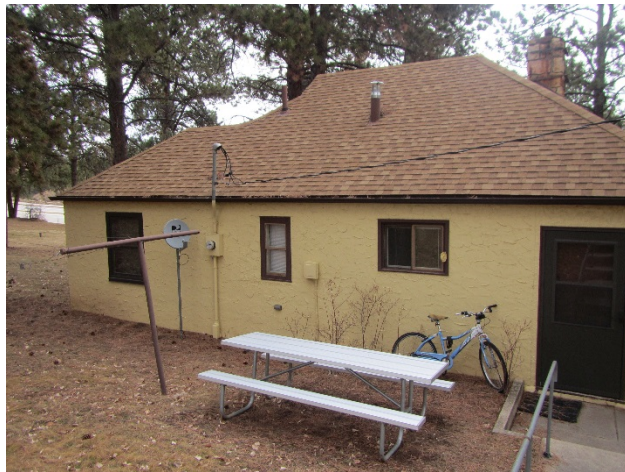
Figure E01. Service conductors at weatherhead on the west side of the house. (HEI 2015)
