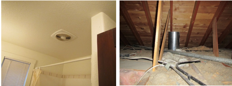
Figure M04. Bathroom – 104, Exhaust fan and termination. (HEI 2015)
