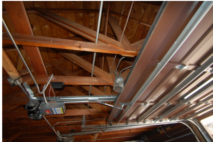
Figure 2-8. Garage 200 Looking at lighting. (SRJA 2015)
