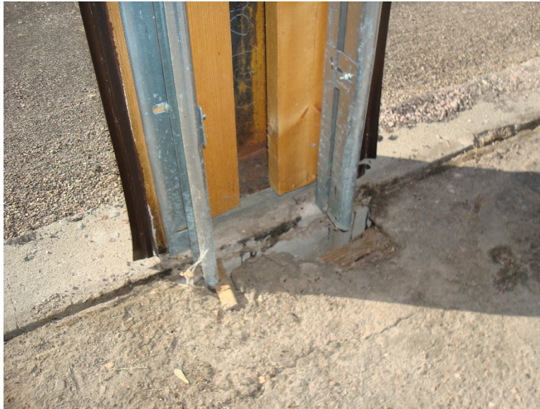
Figure S11. Deteriorated asphalt and wood deck. (SEA 2015)
