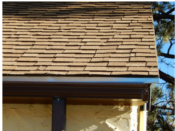
Figure X15. West Elevation detail of south side of the gutter that is short of the roof. (SRJA 2015)
