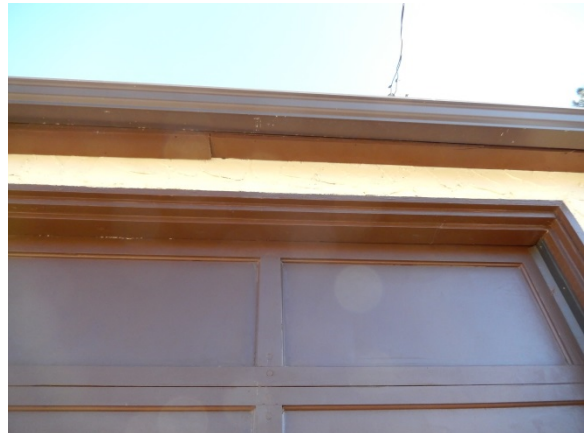
Figure X14. West Elevation detail of loose soffit. (SRJA 2015)
