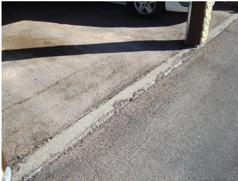
Figure S13. Detail at west foundation wall. Note: the asphalt drive is too high at the edge of the exposed concrete wall. This will not allow for the water to divert away from the building properly. There is no lip or offset at the building entry. Also, the top of the exposed wall is sloping in towards the building. (SEA 2015)
