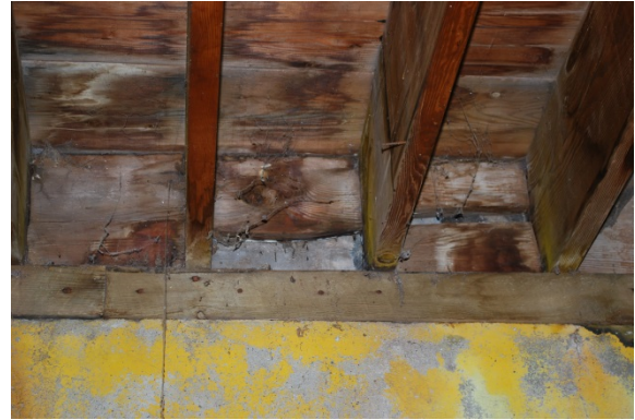
Figure 1-5. Garage 100 Detail of west wall. Note the deteriorated blocking between the joists. (SRJA 2014)
