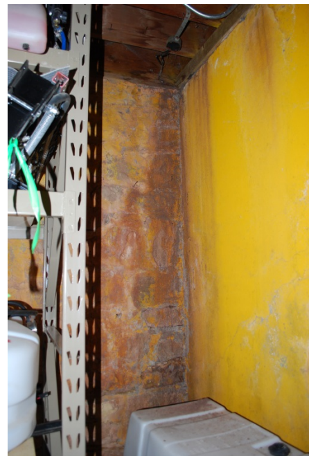
Figure 1-6. Garage 100 Water infiltration in the southwest corner where the south stone foundation wall intersects with the west concrete wall. (SRJA 2014)
