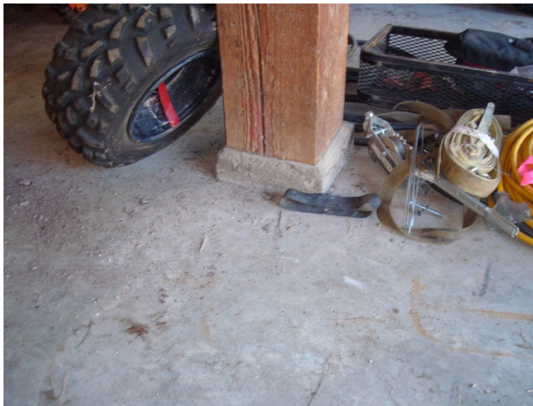
Figure S9. Post bearing on pilaster. (SEA 2015)
