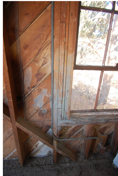
Figure 2-7. Garage 200 Looking at detail of north wall. Note the moisture staining on the interior wood framing and sheathing surfaces. (SRJA 2015)
