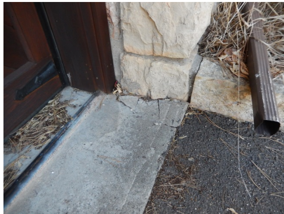
Figure X4. East Elevation detail at the north bay threshold. Note the cracked concrete threshold, the embedded steel threshold and downspout. (SRJA 2015)
