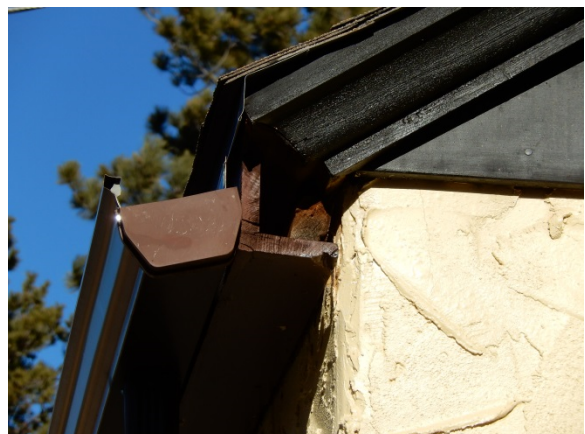
Figure X16. West Elevation detail of the south side of the gutter that is run short of the roof, photograph taken looking north. (SRJA 2015)
