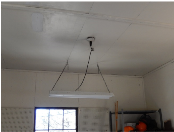
Figure 2-15. Room 201 Ceiling light fixture detail. (SRJA 2014)
