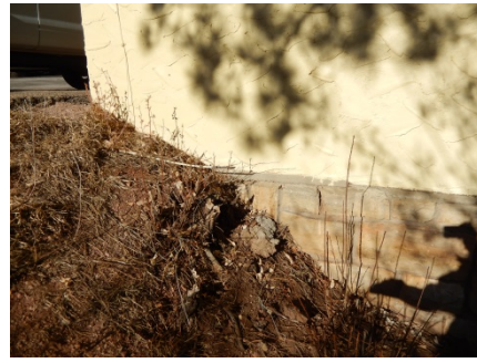
Figure X8. South Elevation detail with grade above the foundation wall in contact with the stucco cladding. (SRJA 2015)
