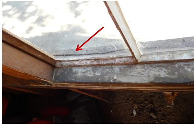
Figure W4. Interior Window 104 detail. Note the missing glazing putty and deteriorated exterior sill. (SRJA 2015)
