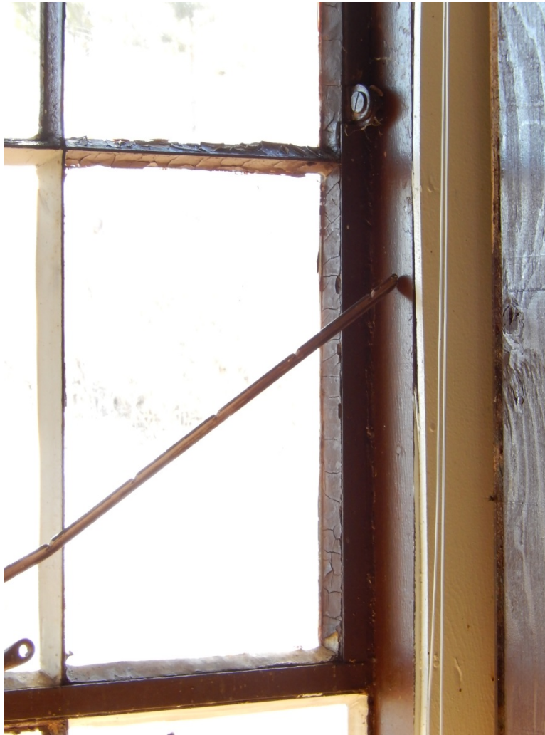
Figure W3. Interior Window 106 detail. Note the deteriorated glazing putty. (SRJA 2015)
