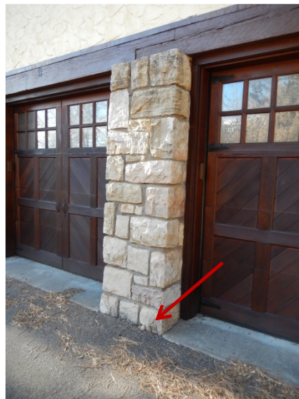
Figure X2. East Elevation detail at stone pier. Note the girder splicing above this pier. The bottom right stone is fractured from the expansion and contraction of the driveway poured directly against the stone. (SRJA 2015)
