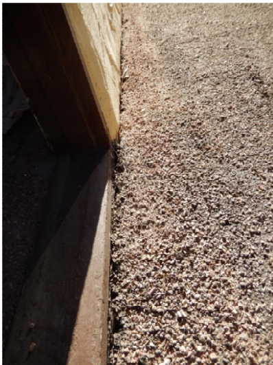
Figure X12. West Elevation detail of joint between asphalt drive and building. There is no soft joint installed. (SRJA 2015)
