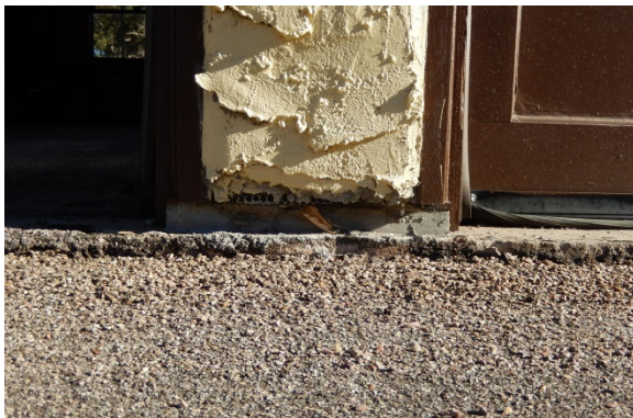
Figure X13. West Elevation detail of missing stucco at base of pier and exposed wire lath. (SRJA 2015)
