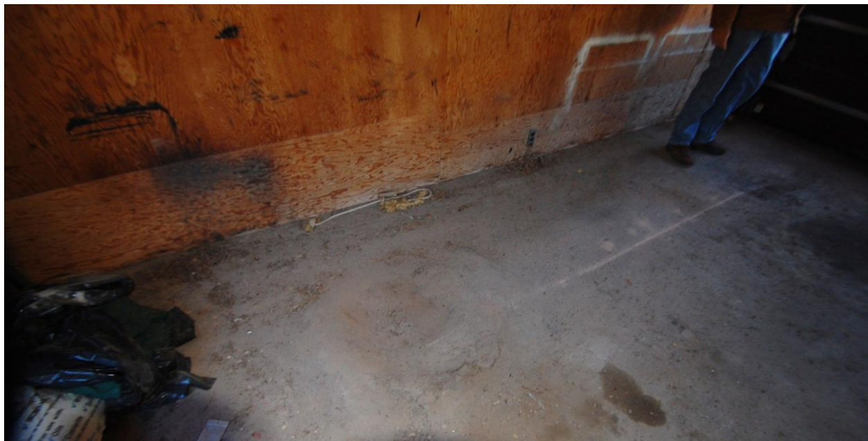
Figure 2-9. Garage 200 Looking at deep depression in the asphalt in the south garage bay. (SRJA 2015)
