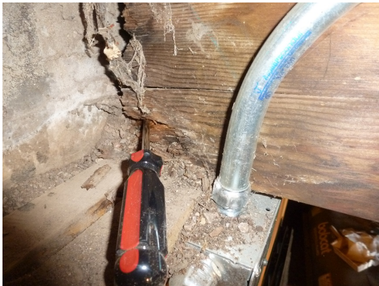
Figure S14. Deteriorated joist end at west foundation wall. (SEA 2015)
