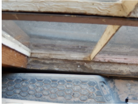
Figure W2. Window 103 Detail with truck bumper against window frame. Note the deteriorated wood sill on the exterior of the window. (SRJA 2015)
