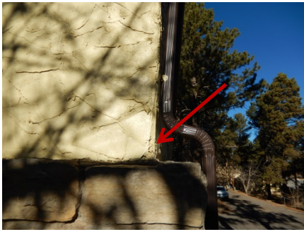
Figure X7. South Elevation detail at southeast corner where missing stucco has exposed metal lath. (SRJA 2015)
