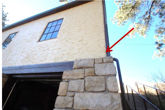
Figure X3. East Elevation detail at northeast corner. Note the stucco crack at the corner. (SRJA 2015)
