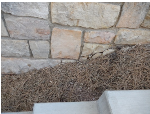
Figure X19. North Elevation stone foundation deterioration detail. (SRJA 2014)
