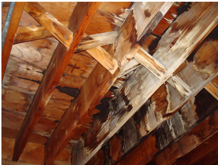
Figure S10. Asphalt stained floor joists. (SEA 2015)
