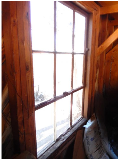
Figure W1. Interior window detail. Note the missing glazing putty. (SRJA 2015)
