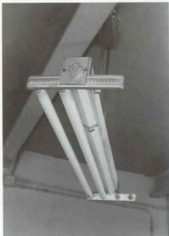
Fig. 45. Room 205 (Records Office), Light Fixture Type FL-C [1988].
